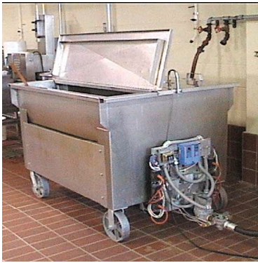
Gas-fired cook/steep tank for Grain Nixtamalization
